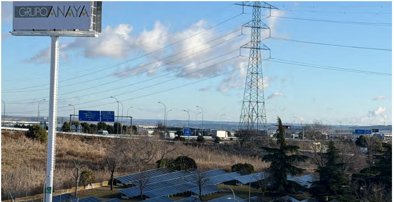
Installation of solar panels at the logistics site in Getafe, Spain (Grupo Anaya).
